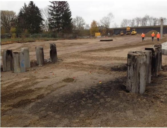
Figure 7: Construction of the bridge – installation of piles for one of the middle foundation
